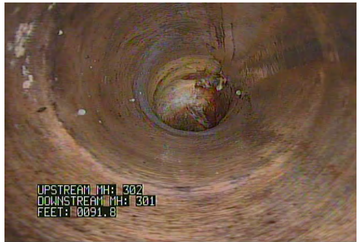
TF - Tap, Factory Made @ 91.8 ft. T LINER (CIPP)
