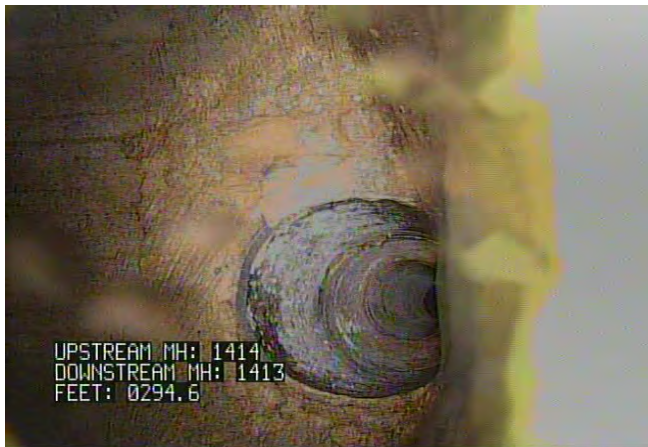
TFA - Tap, Factory Made: Active @ 294.6 ft. LATERAL INSIDE THE MH (DYE PRESENT)
