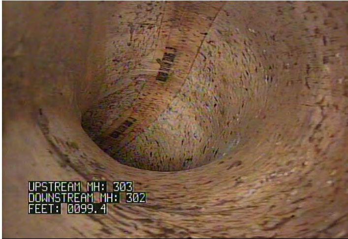
TF - Tap, Factory Made @ 99.4 ft. T LINER (CIPP)
