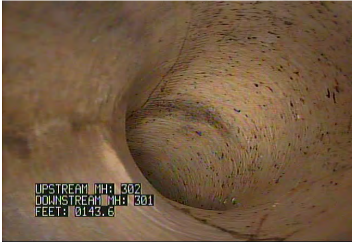
TF - Tap, Factory Made @ 143.6 ft. T LINER (CIPP)
