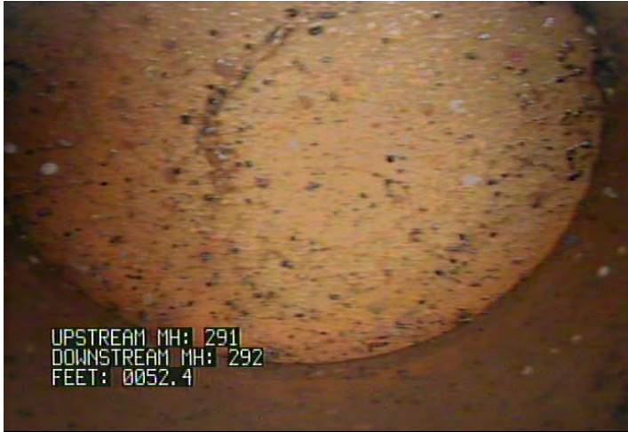
TFC - Tap, Factory Made: Capped @ 52.4 ft.
