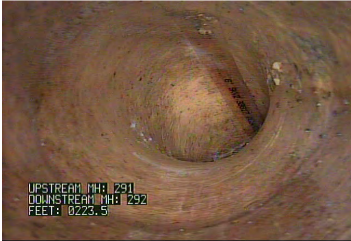
TF - Tap, Factory Made @ 223.5 ft. T LINER (CIPP)
