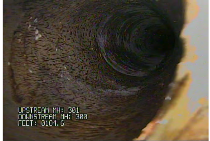
TF - Tap, Factory Made @ 184.6 ft. T LINER (CIPP)
