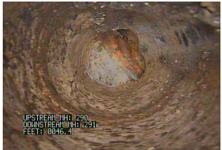
TF - Tap, Factory Made @ 46.4 ft. T LINER (CIPP)
