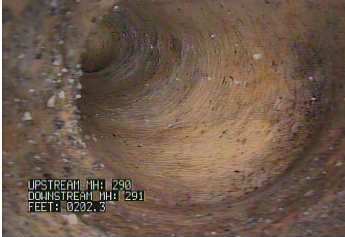
TF - Tap, Factory Made @ 202.3 ft. T LINER (CIPP)
