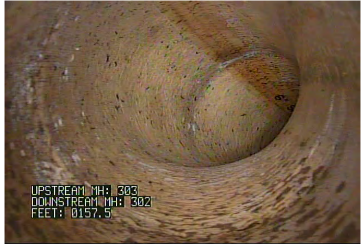
TF - Tap, Factory Made @ 157.5 ft. T LINER (CIPP)
