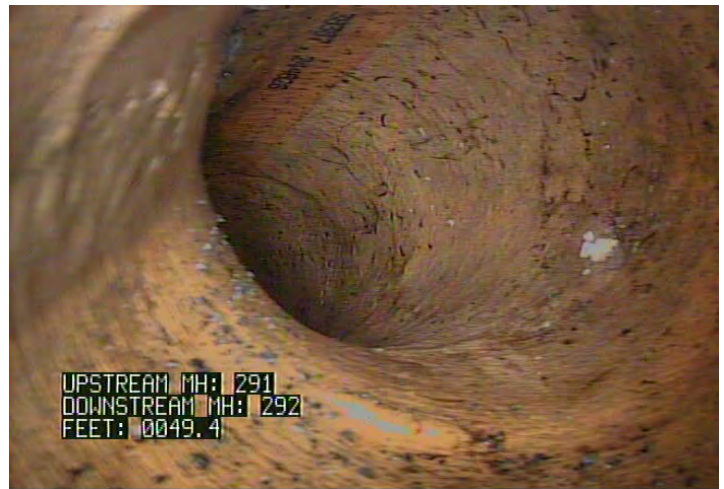
TF - Tap, Factory Made @ 49.4 ft. T LINER (CIPP)
