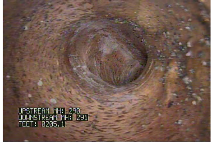
TF - Tap, Factory Made @ 205.1 ft. T LINER (CIPP)
