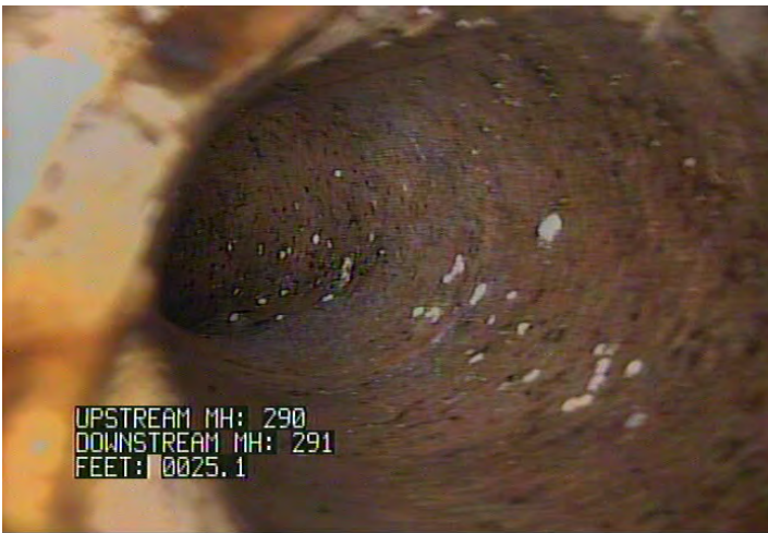
TF - Tap, Factory Made @ 25.1 ft. T LINER (CIPP)
