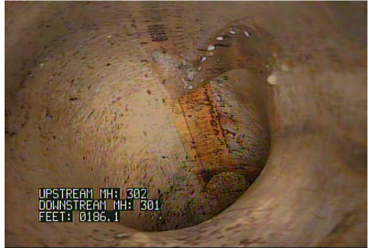
TF - Tap, Factory Made @ 186.1 ft. T LINER (CIPP)
