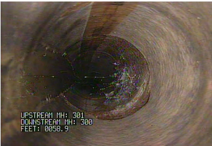
TF - Tap, Factory Made @ 58.9 ft. T LINER (CIPP)
