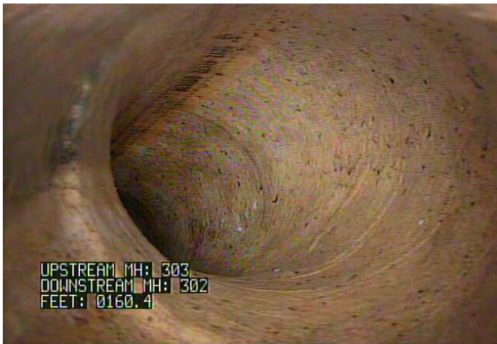
TF - Tap, Factory Made @ 160.4 ft. T LINER (CIPP)
