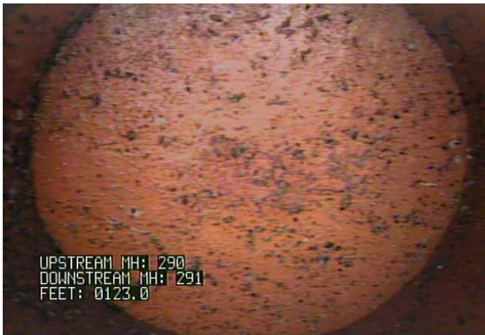
TFC - Tap, Factory Made: Capped @ 123.0 ft.
