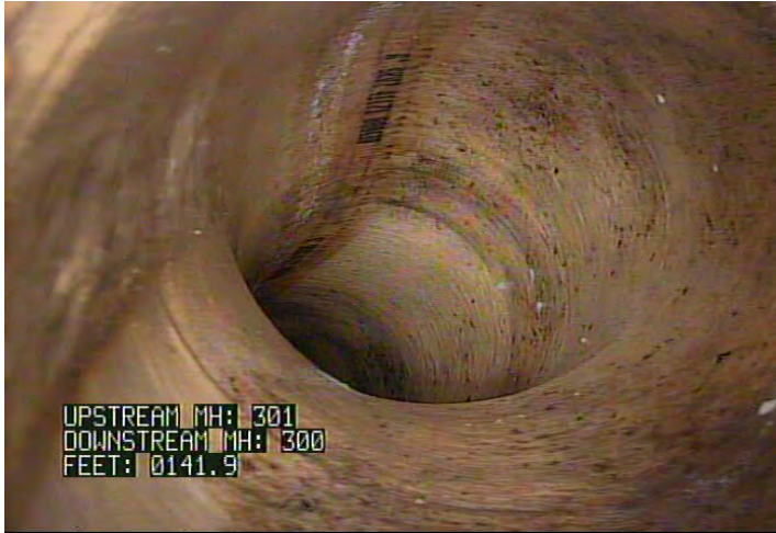
TF - Tap, Factory Made @ 141.9 ft. T LINER (CIPP)
