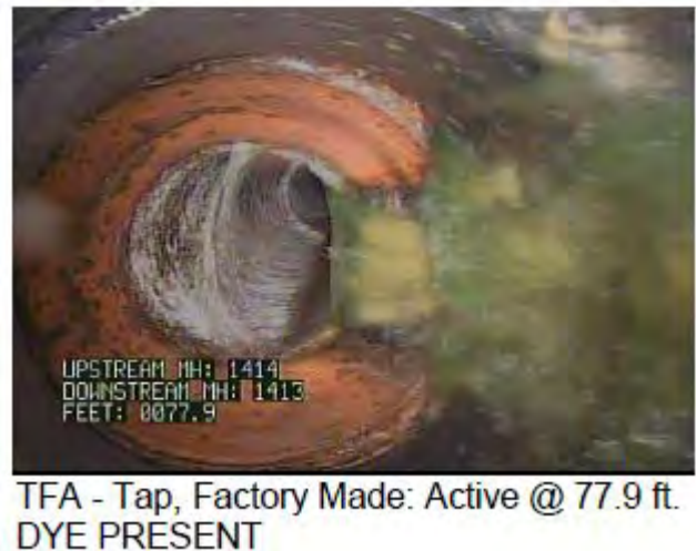
Figure 3.11 Private Property Lateral showing I/I from Dye Water Test
