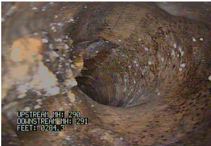
TF - Tap, Factory Made @ 284.3 ft. T LINER (CIPP)
