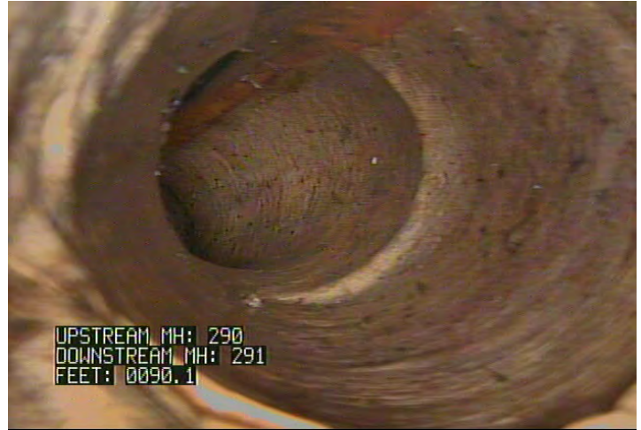
TF - Tap, Factory Made @ 90.1 ft. T LINER (CIPP)
